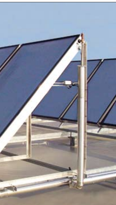
Interesting for Italy: Weishaupt's versions K3 and K4 of the large-sized solar system WTS-F1 Photo: Weishaupt
